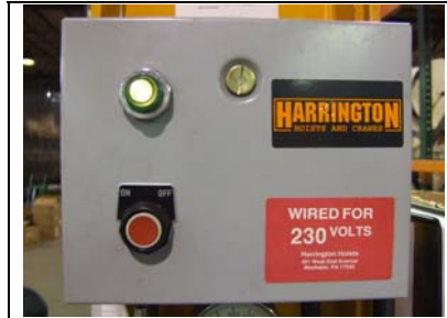
Figure 4 – DHLT Control Panel
